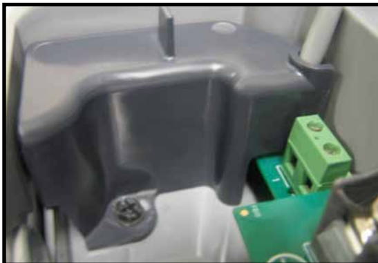
Figure 15: Plastic Cover Installed In Terminal Box
